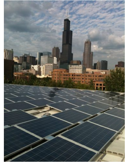
Figure 4. Rooftop Solar Installations Rooftop solar installation on Douglas Hall at the University of Illinois at Chicago has no effect on land resources, while producing electricity with zero emissions. Source: Office of Sustainability, UIC
